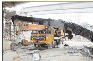
SRINAGAR, JAN 31: A girder fell while it was being lifted by crane to be
